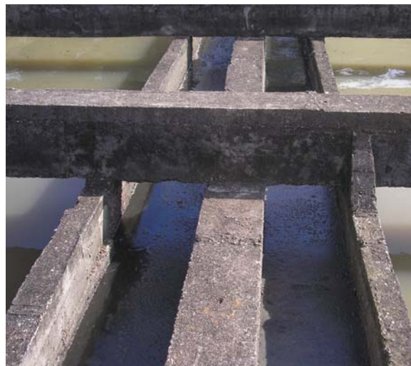
Figure 13 Scum Chamber Filled with Digested Solids
